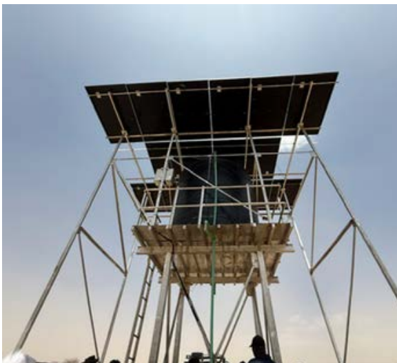
Solar powered electric well. Pumps enough water for the village, the surrounding area and their animals.
